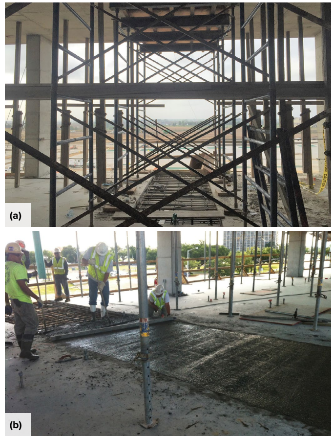
Fig. 1: Pour strips are gaps in floor structures designed to minimize restraint of early stage volume changes of concrete: (a) backshoring and changes in elevation create logistical and scheduling issues; and (b) delayed concrete placements result in high unit costs
